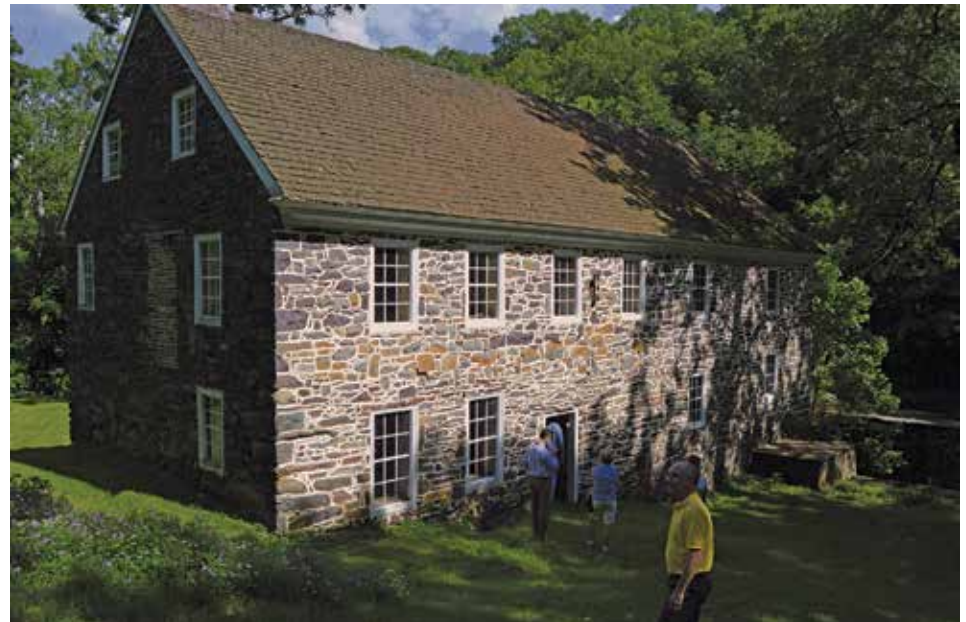
The western portion of the Sunrise Mill was repainted a few years ago, but significant restoration is still needed.
