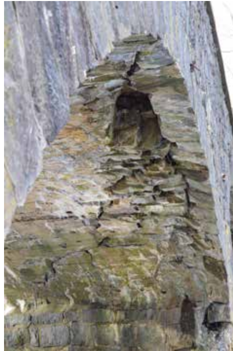
Failing arch on the Old Gravel Pike Bridge.
