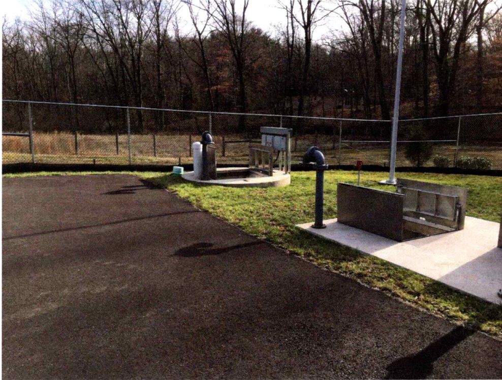
1 Pump Station #20 – Wet Well Exterior.
