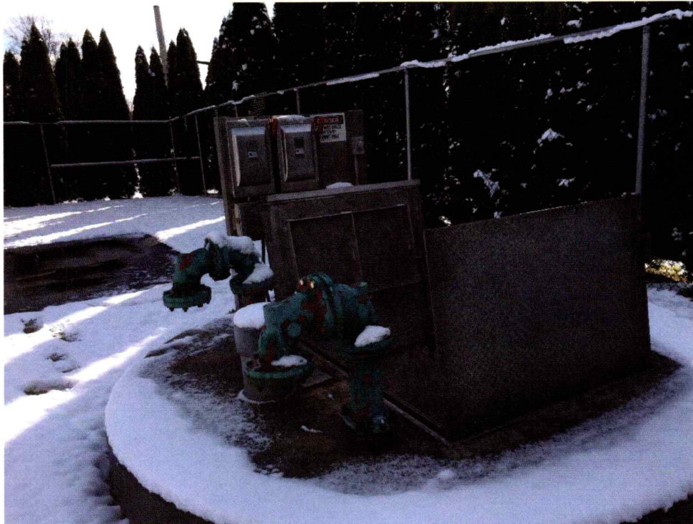
3 Pump Station #19 – Wet Well Exterior.
