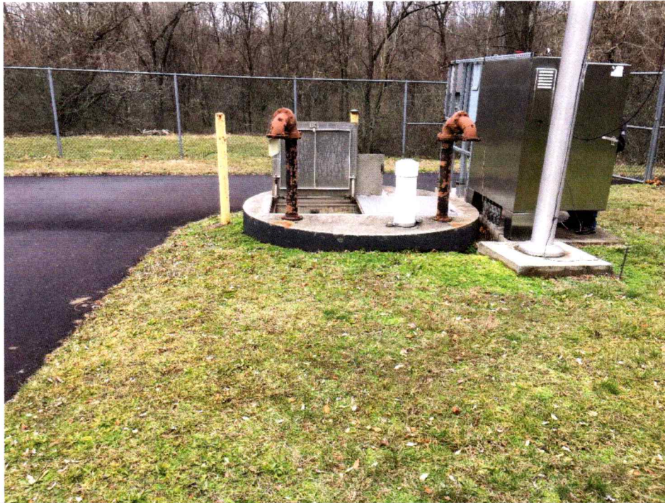
3 Pump Station #16 – Wet Well Exterior.
