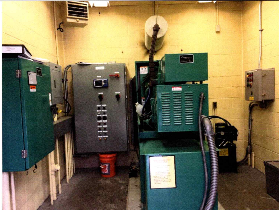
4 Pump Station #4 – Building Interior
