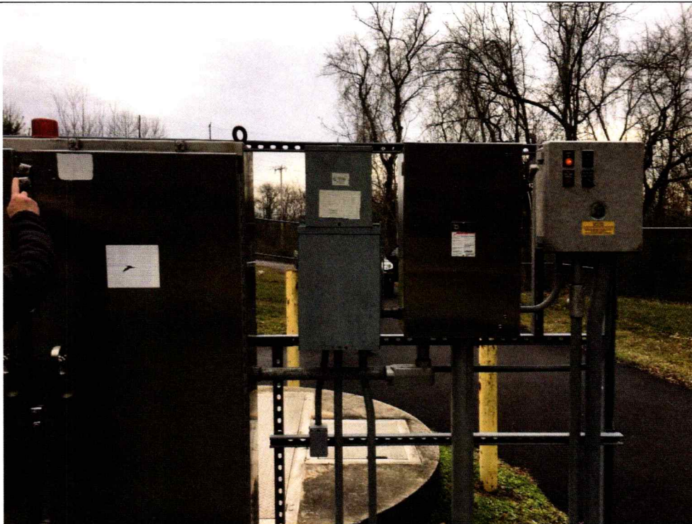
4 Pump Station #16 – Control Panel.
