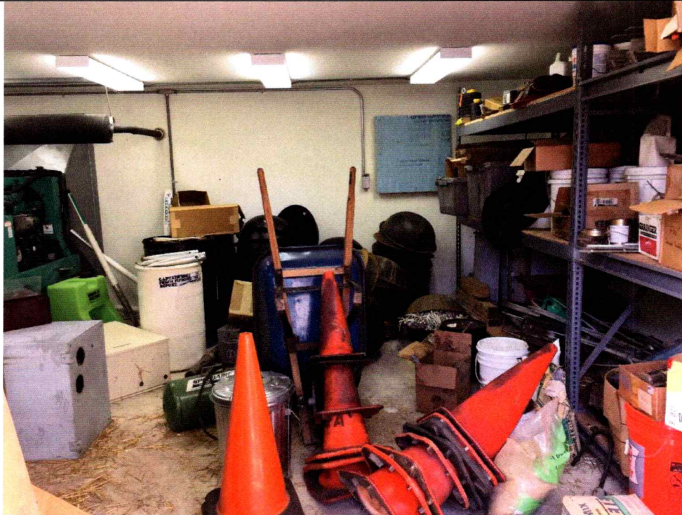
2 Pump Station #8 – Building Interior.
