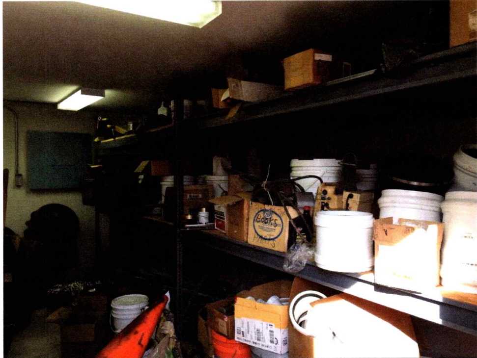
3 Pump Station #8 – Building Interior.
