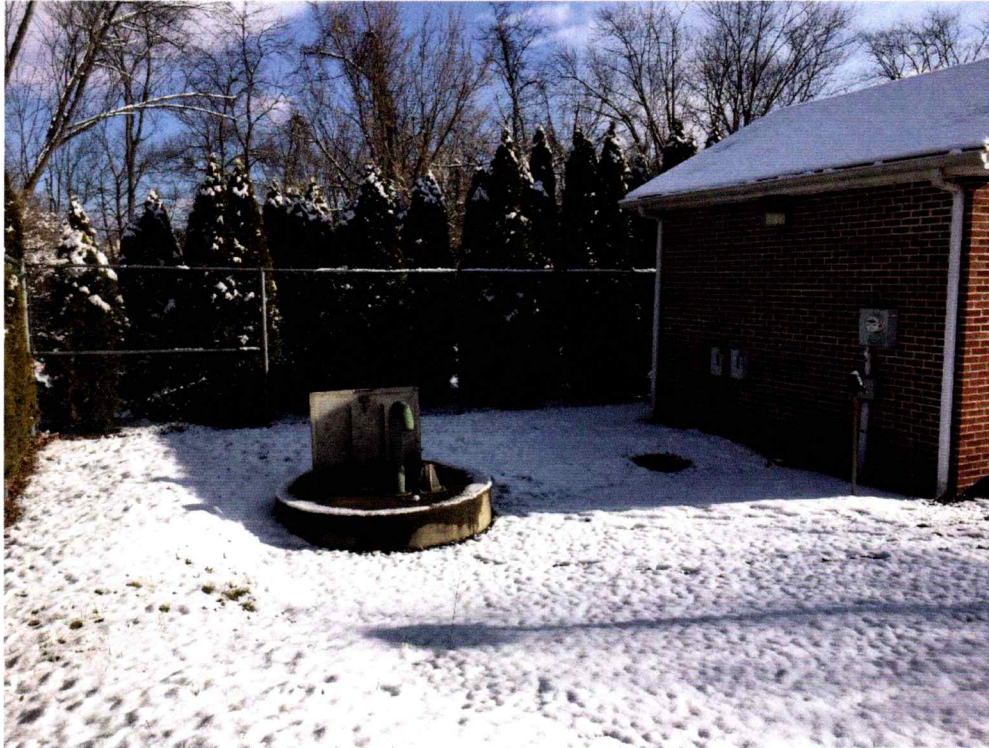
1 Pump Station #15 – Wet Well Exterior.
