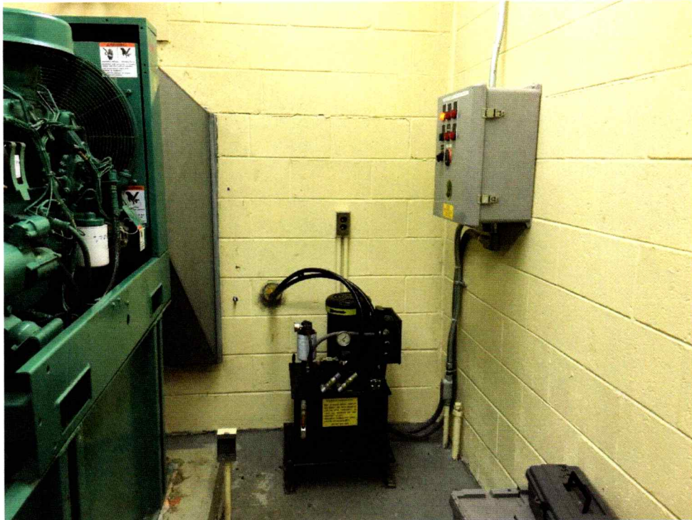
3 Pump Station #4 – Building Interior
