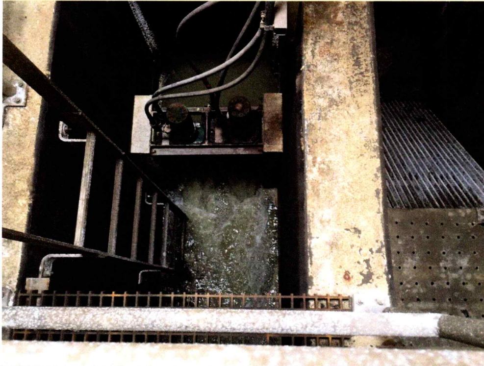
7 Pump Station #6 – Wet Well
