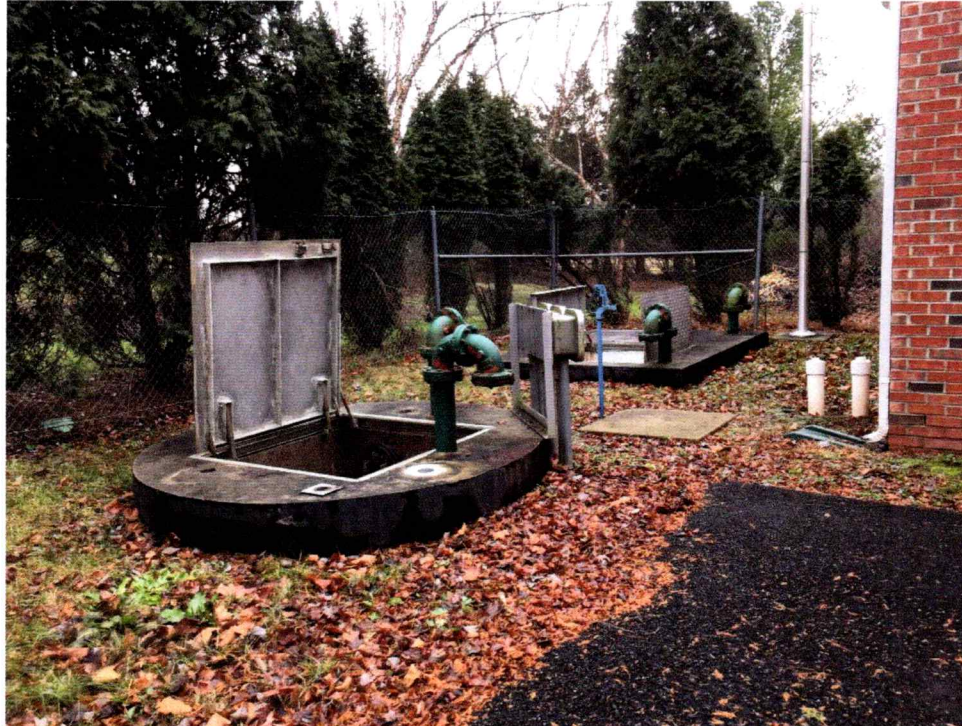
1 Pump Station #14 – Wet Well Exterior.
