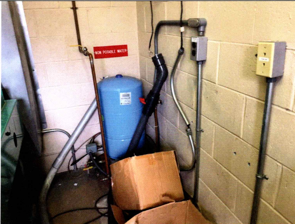
4 Pump Station #9 –Building Interior.
