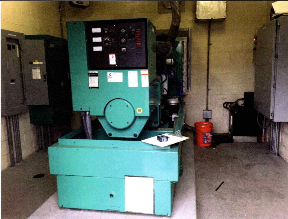
4 Pump Station #12 – Building Interior
