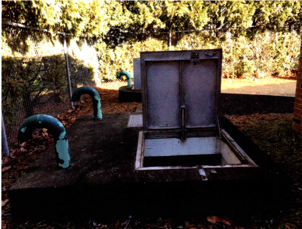
1 Pump Station #13 – Wet Well Exterior.
