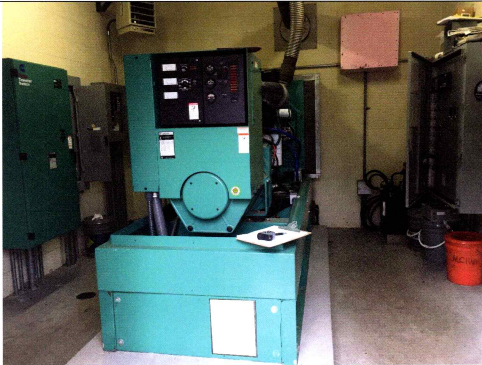
4 Pump Station #14 – Building Interior.
