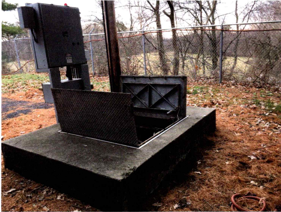
3 Pump Station #7 – Wet Well Exterior.
