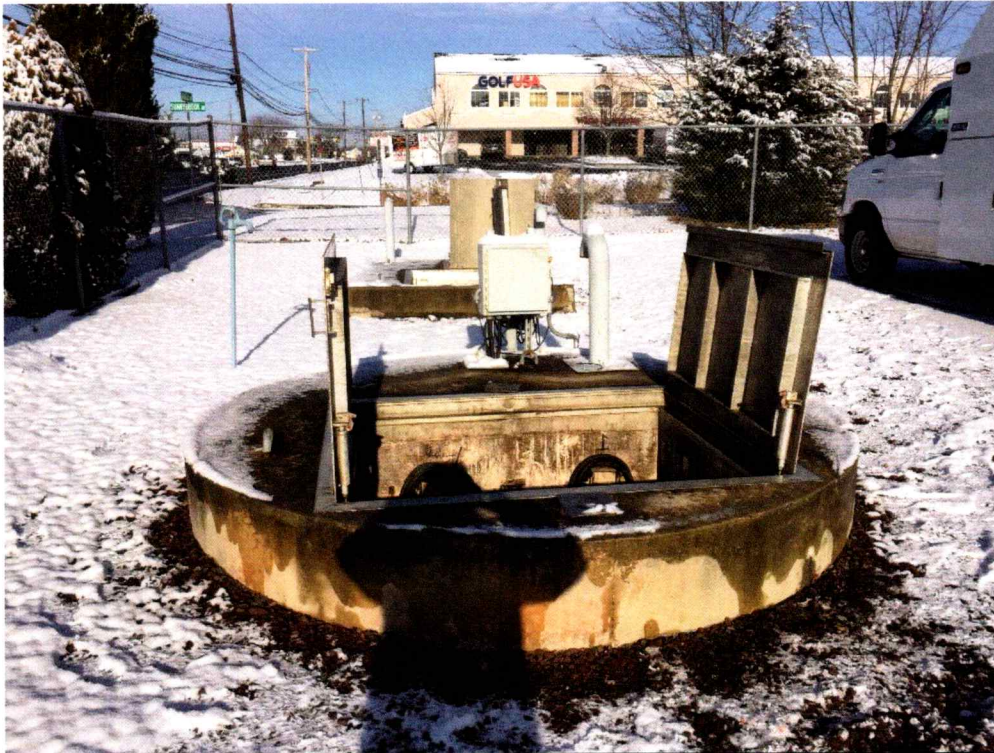
1 Pump Station #10 – Wet Well Exterior.
