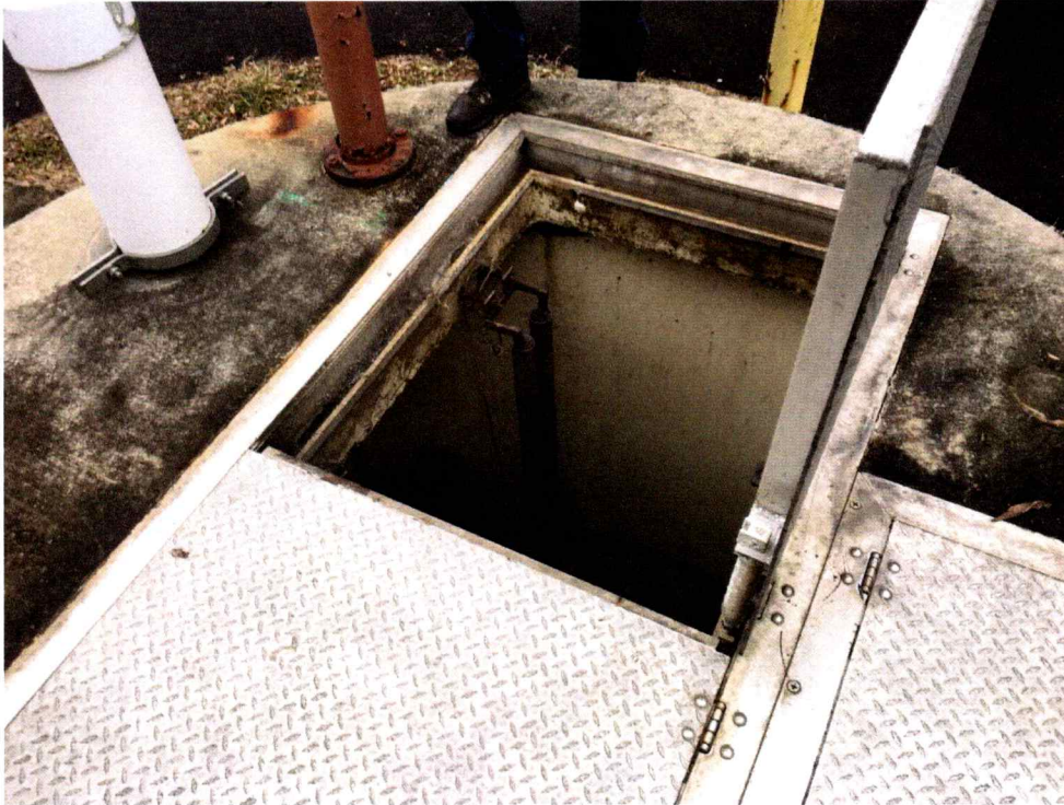
3 Pump Station #17 – Wet Well Exterior.
