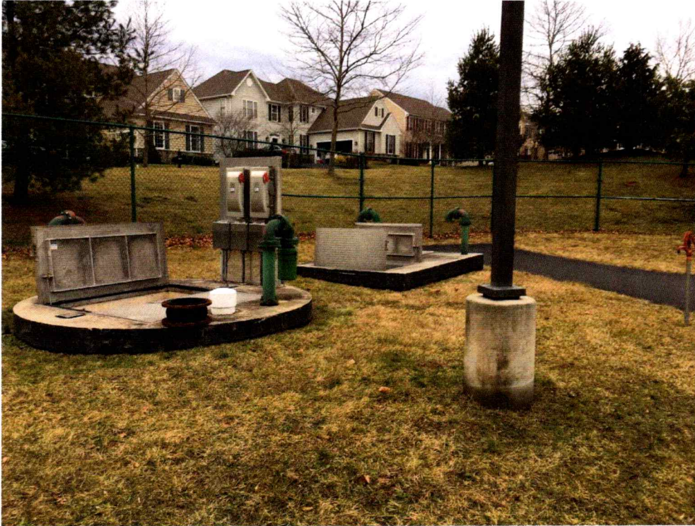
1 Pump Station #18 – Wet Well Exterior.
