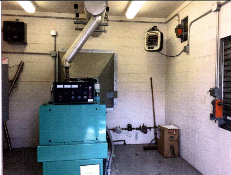
4 Pump Station #15 – Building Interior.
