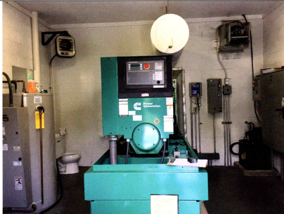
4 Pump Station #19 – Building Interior.
