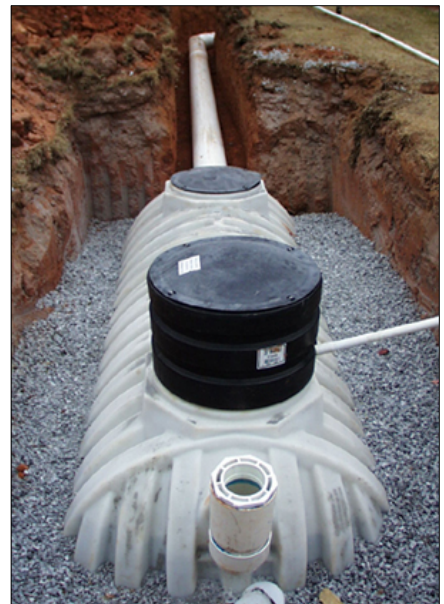
Rain harvesting systems collect rain from roof tops, air conditioning units and even refrigerators. The water is stored underground in a cistern, like this one that holds more than 1,000 gallons.
